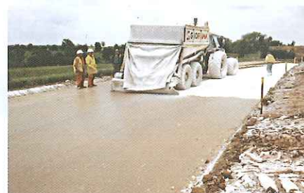
Road construction work on the A429 using University of Glamorgan's soil stabilisation technology
